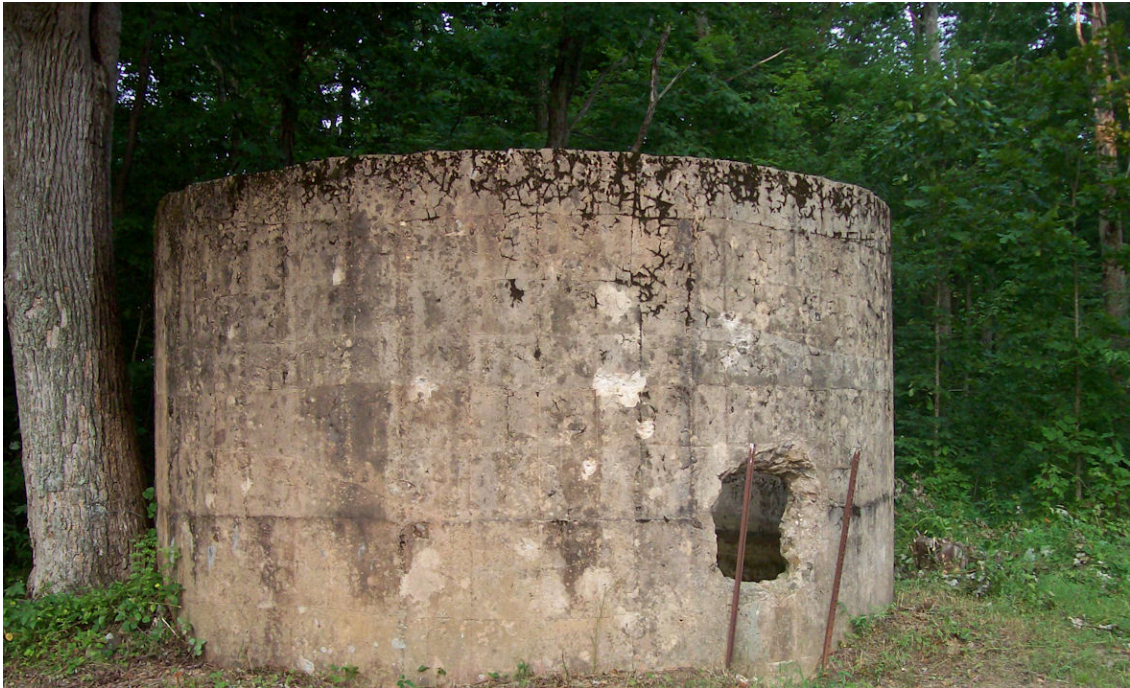
A view showing how a hole was knocked in the side of the cistern to allow local women to get water for washing clothes and other chores. This happened after the hotel burned and the place was abandoned
