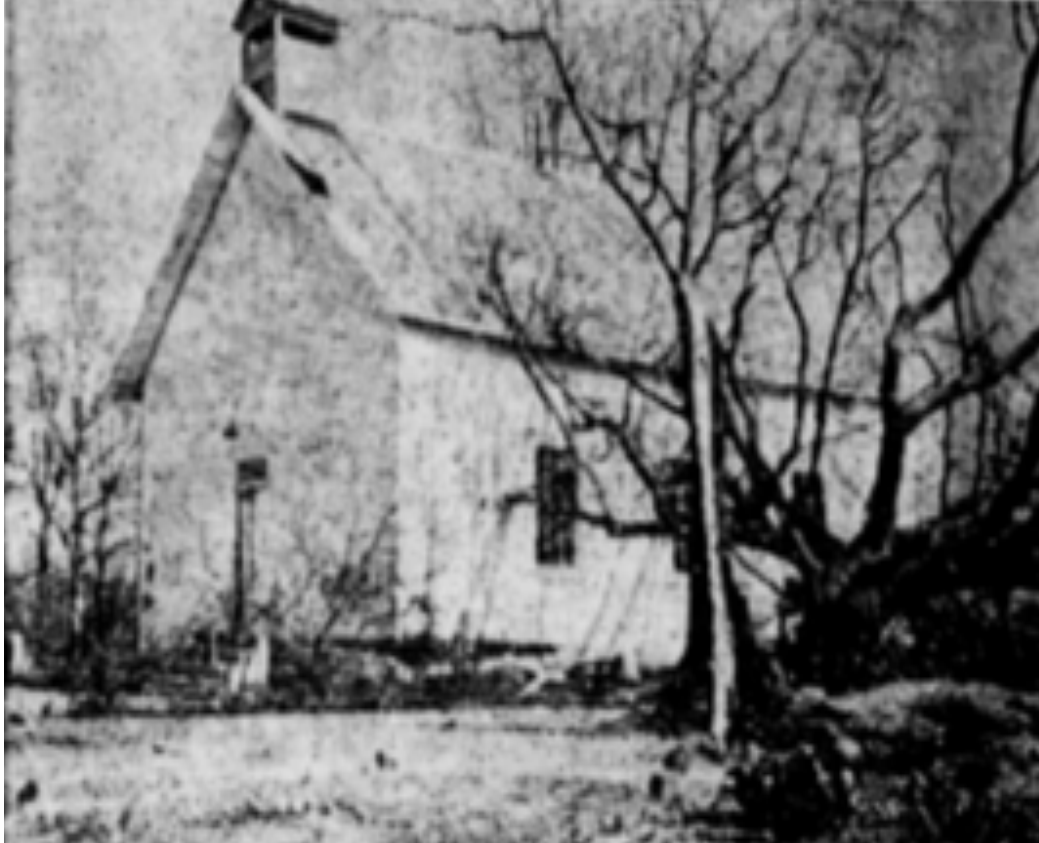
Hobbs' Hill Methodist Church on Feb. 14, 1952 after a tornadic wind forced a large tree into the building moving it off its foundation
