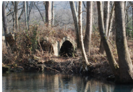
Two stone arches from of the Elkhead River Bridge on the east side of the river are barely visible through the brush.
