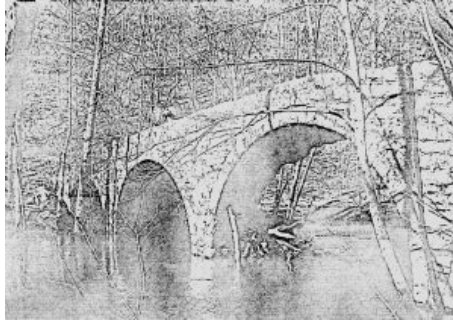
The Elkhead River Bridge as it looked in 1977. (The image is a scan of an email of a PDF page from a printed document.)
