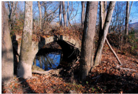
Although the area is overgrown and littered with brush, the site of the old bridge is a historic and potentially beautiful spot.
