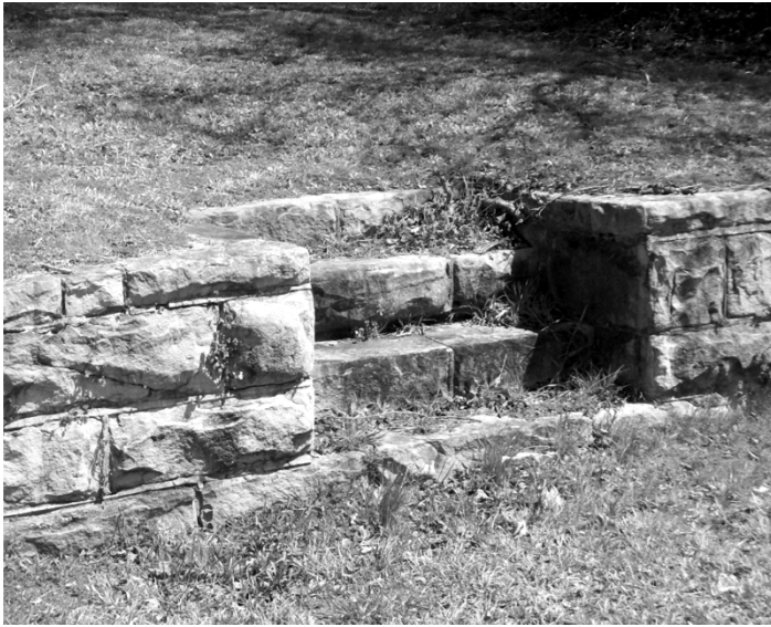
Above: four steps previously leading up from Depot Street to the Warren Memorial Cumberland Presbyterian Church Building
