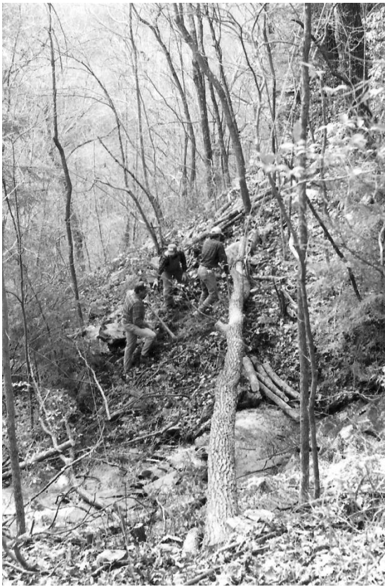
Grady Ward Partin and Curt Partin built a tramway to move rock for use in their landscaping business. The work began.
