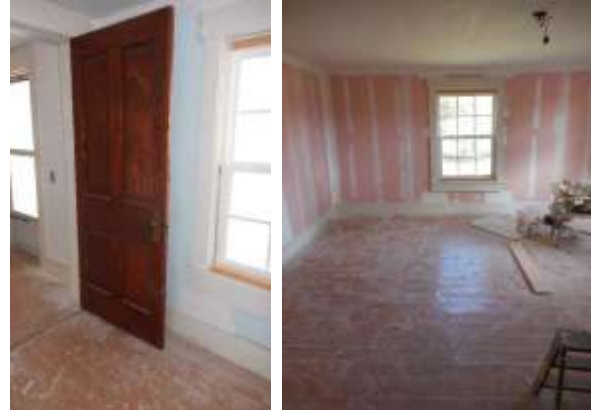
Figure 9. One of the bedrooms on the upper level as it undergoes renovation.
